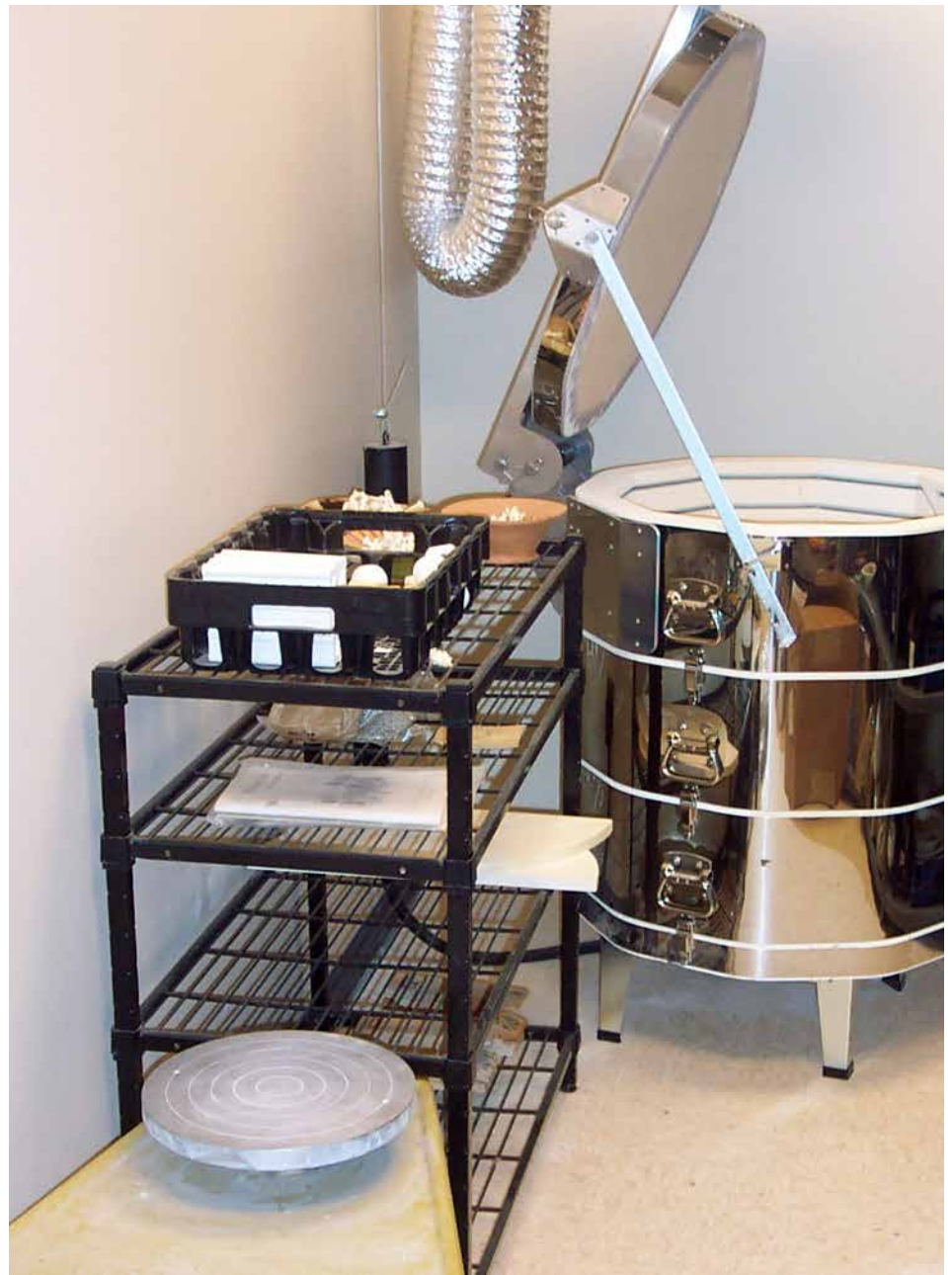
Figure 1 Kiln Room with Appropriate Ventilation
